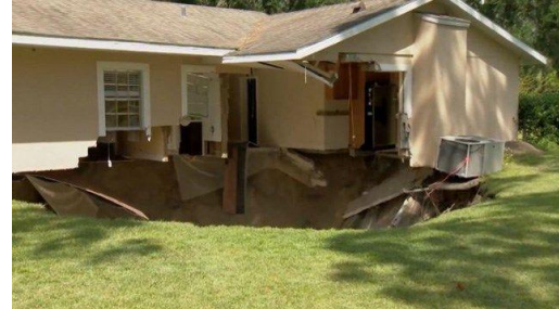
(b) Sinkhole effect of a house in Florida
